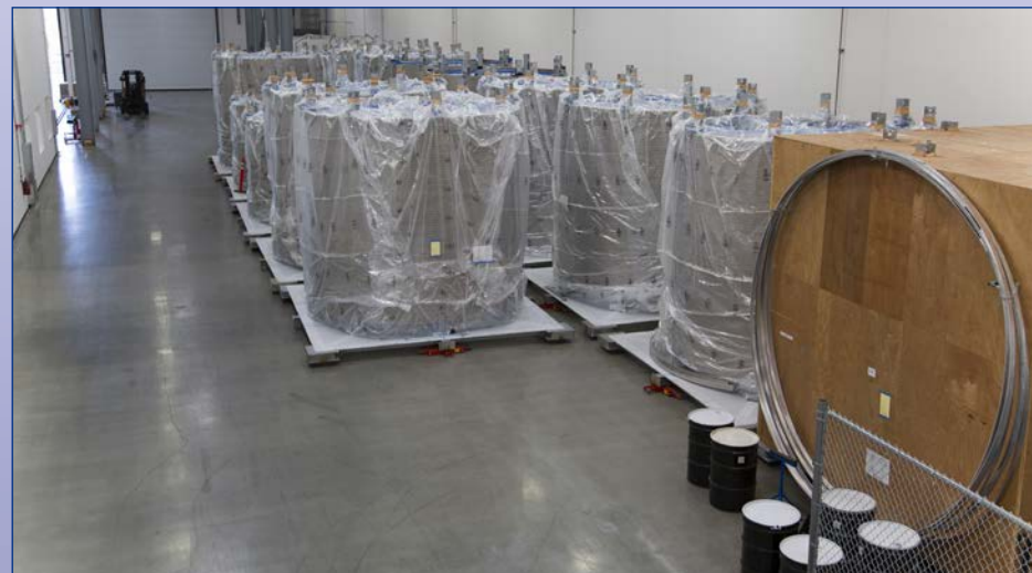
Conductor spools stored prior to winding
