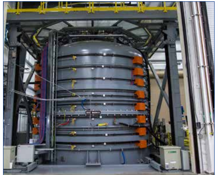
Furnace closed for module heat treatment
