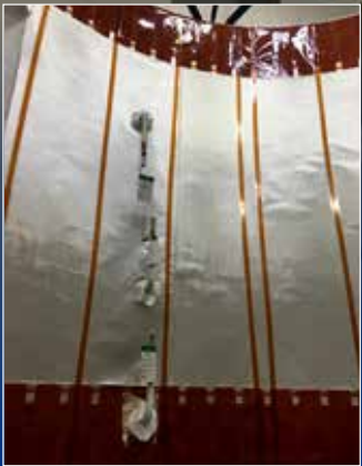
Helium inlet pipe with ground insulation
