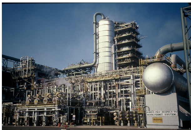
Figure 2. Gulftronic electrostatic separator and RFCC unit.
